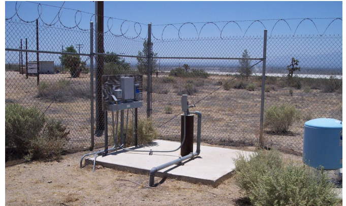
Tank system at El Mirage OHV Area
