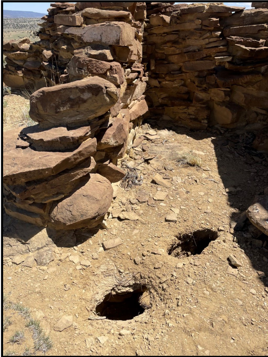
Figure 6: Natural collapse features were noted during monitoring near the defensive wall of Big Bead Mesa NHL
