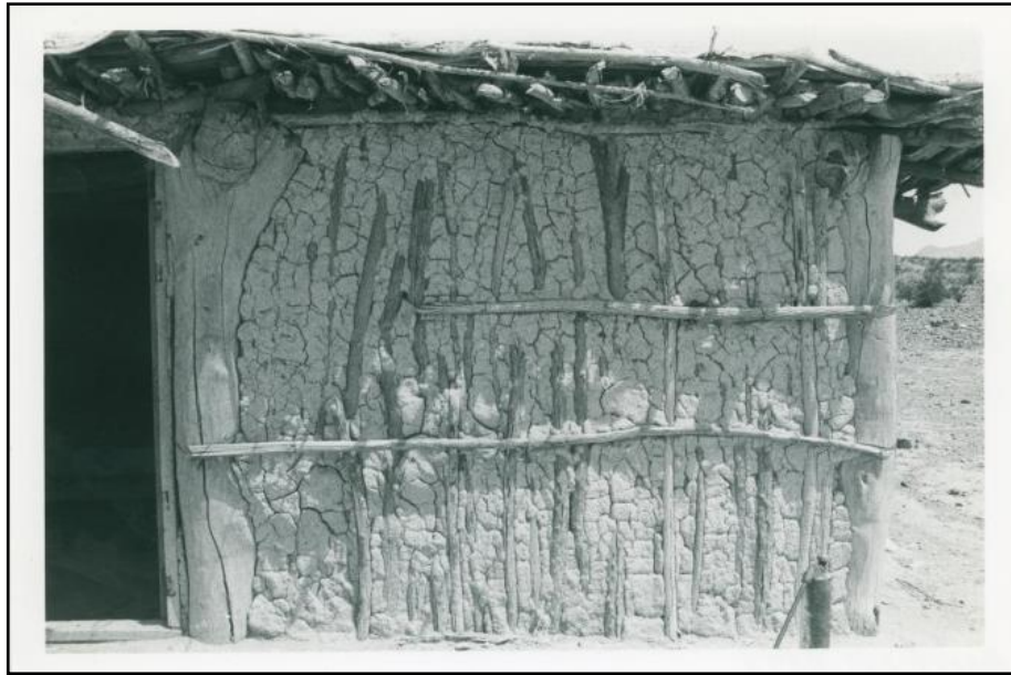
Figure 4. Historic jacal House in Ojinaga, Chihuahua, Mexico. The Merchant Site Rooms may have been constructed in a similar manner (Photograph credit Rescuing Texas History 2016 Archive, Texas A&M University, Kingsville).
