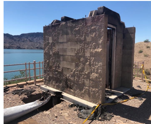
One of 3 vandalized shoreline vault toilets in 2023.
