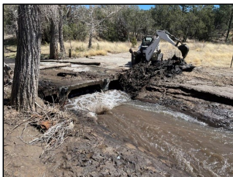
A small excavator removes debris and silt from a low water crossing after a rain event.
