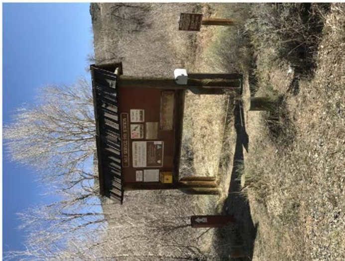
Aged Kiosk Needing Replaced
