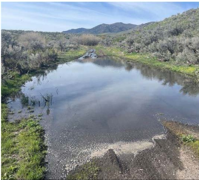
Flooded access road being widened by the public.
