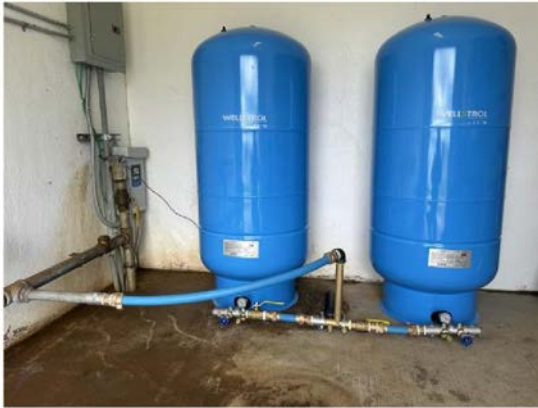
New Hydro-pneumatic Tanks installed
