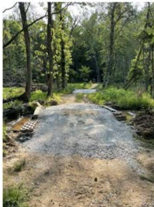
Culverts at Thompson Creek Loop
