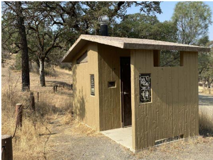
Vault toilet needing facility repair
