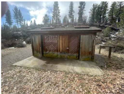
Photo of Bizz Johnson Vault to be replaced
