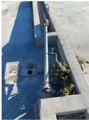
Broken Hose Tower
