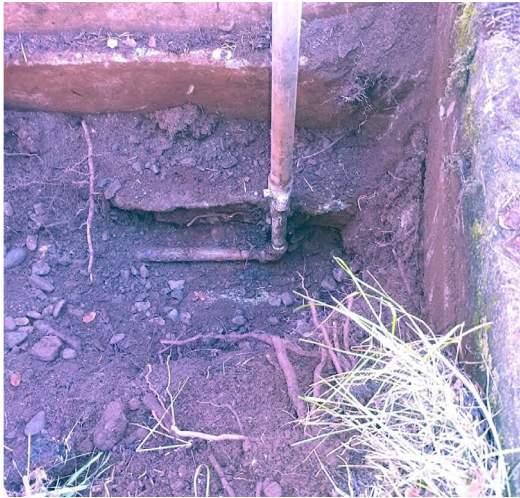
Broken Water Line in Hyatt Lake Campground
