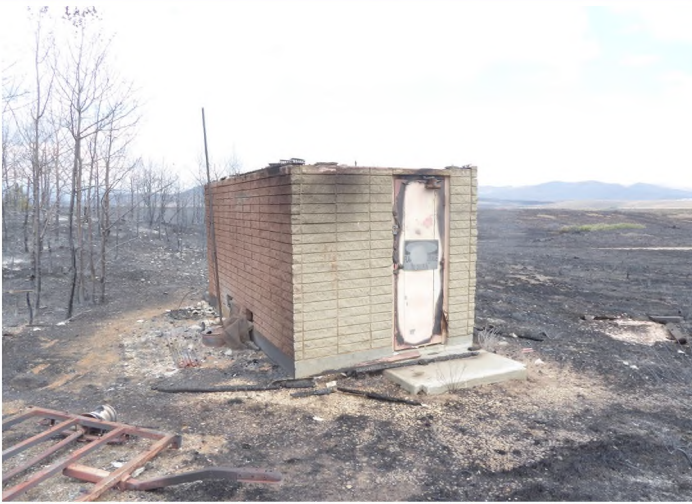
Wildhorse burned vault toilet
