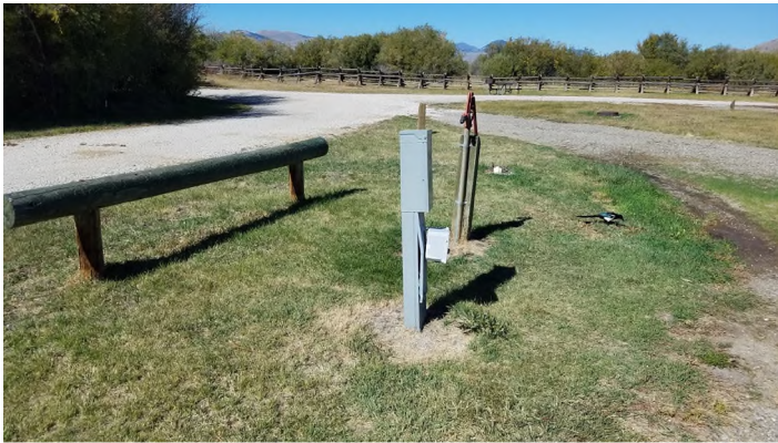
Broken electrical pedestal.
