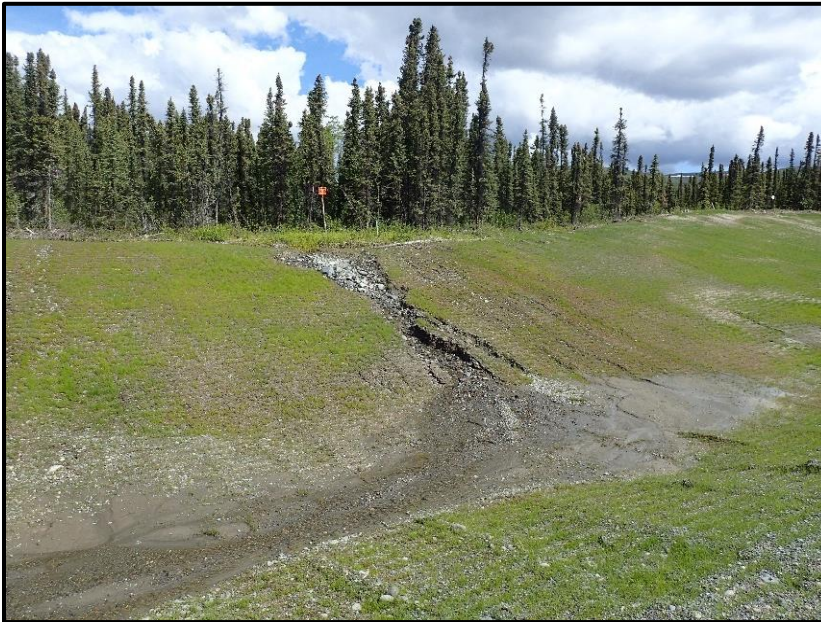
Figure 58. Gully erosion on a freshly graded hillslope.
