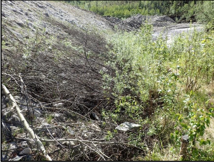
Figure 46. Brush mattress placed at the transition from the bankfull bench and the hillslope. Cuttings extend into the ground to a depth that is equal to the water table.
