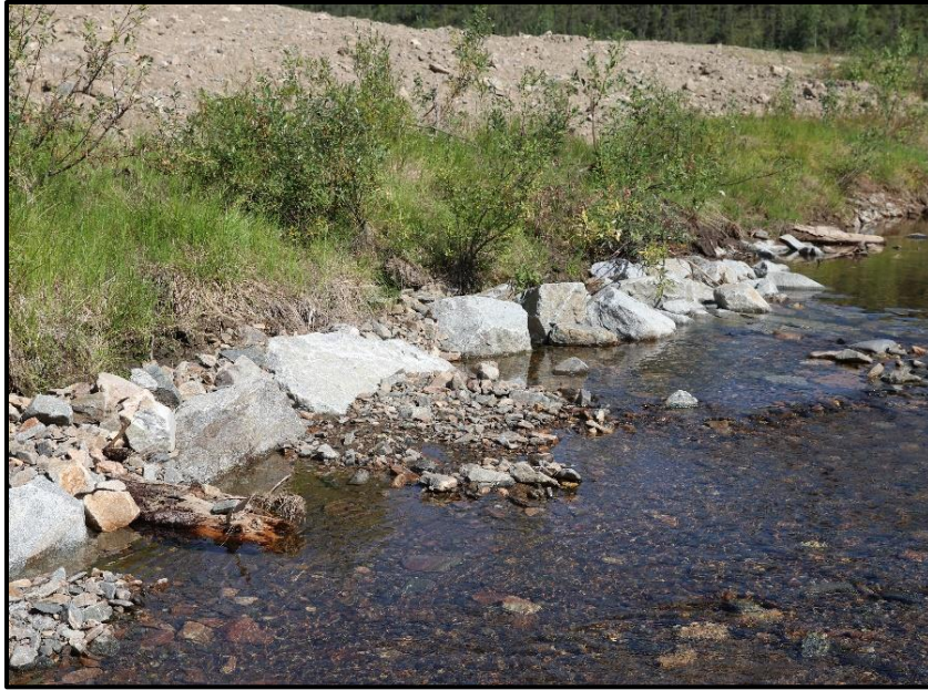
Figure 41. Toe protection using boulders and no wood. This is less desirable than a mixture of wood and boulders.
