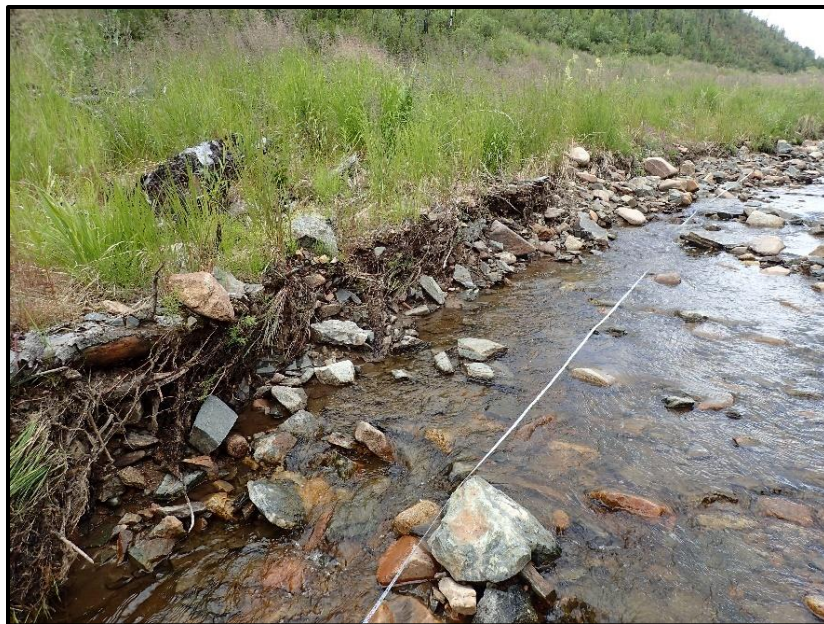
Figure 67. Minor bank erosion.
