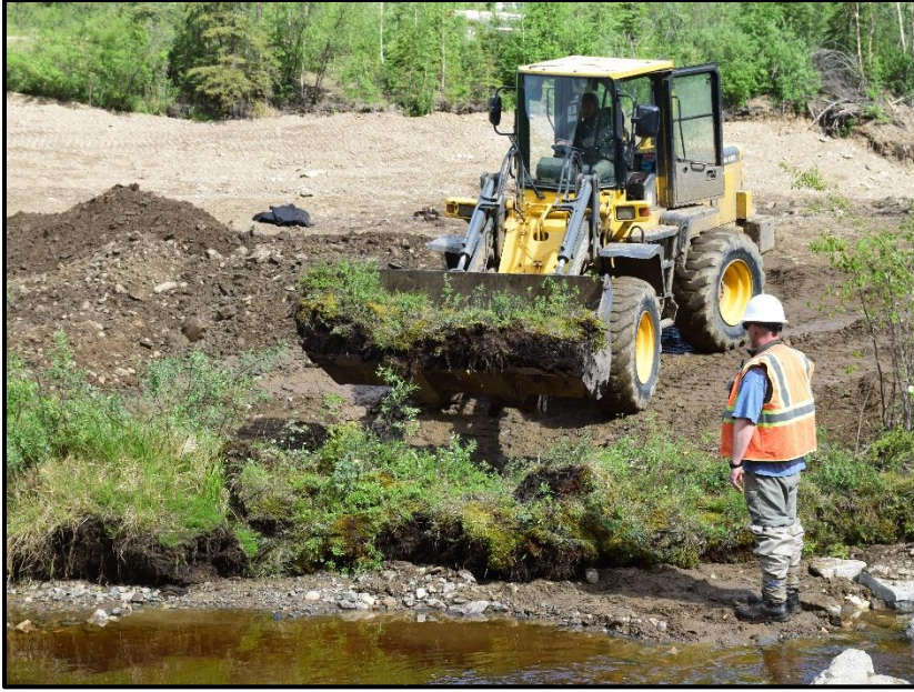
Figure 43. Transplanting with a wheel-loader. After the transplants are placed, a track hoe is used to finalize their placement, cover the seams, and to meet grade requirements.
