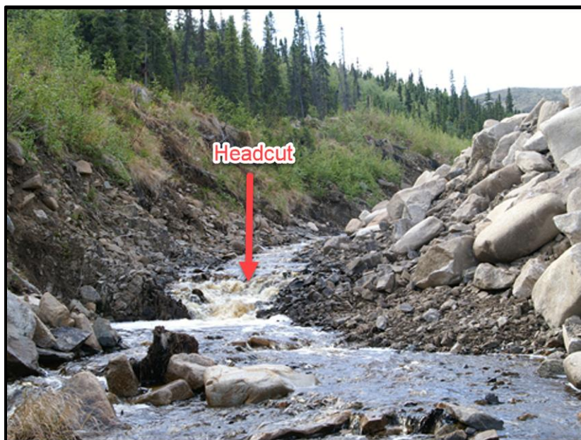
Figure 18. G stream type used for reclamation resulting in bed erosion (headcut).
