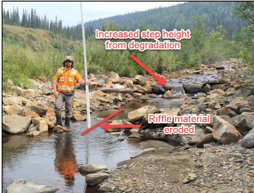
Figure 59. Degradation failure of a constructed riffle (structure failure).
