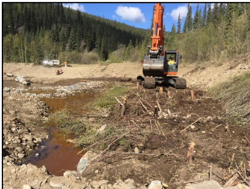
Figure 38. A bankfull bench being constructed. Toe wood is used to stabilize the bottom (toe) of the bank, Transplants are used to stabilize the remainder of the bank and the bench.
