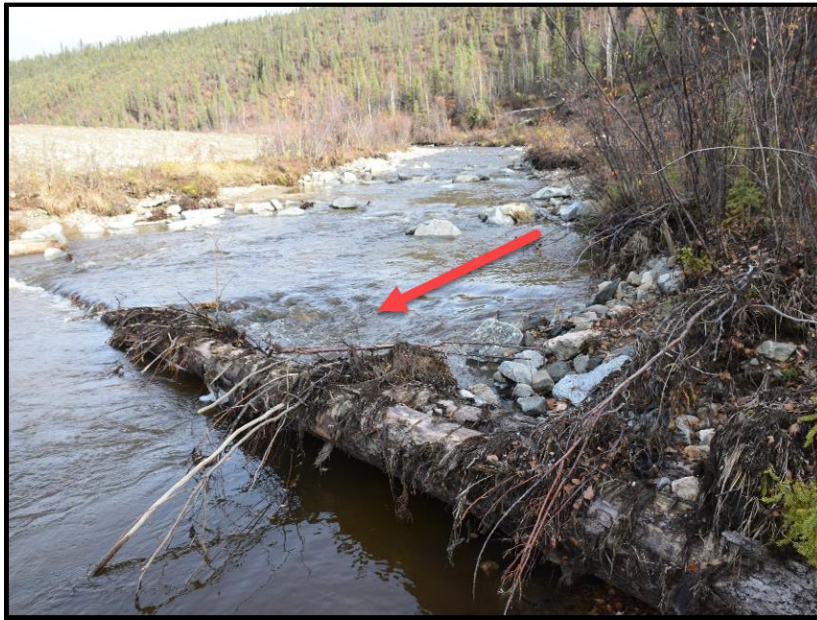
Figure 60. Log roller structure failure.
