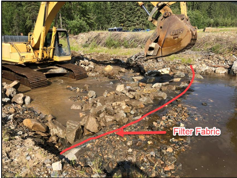
Figure 35. Boulder sill with filter fabric being constructed at the head of a constructed riffle.
