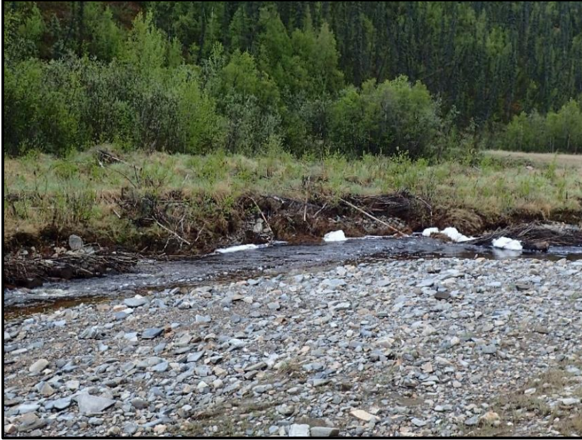
Figure 57. Bank erosion of concern. Loss of toe wood and streambank transplants in a meander bend.
