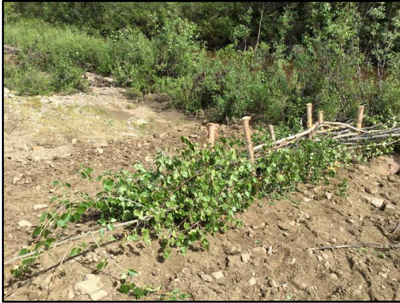
Figure 52. Brush bar installed by hand on a section of bankfull bench devoid of vegetation. This technique was used due to the low supply of transplants.
