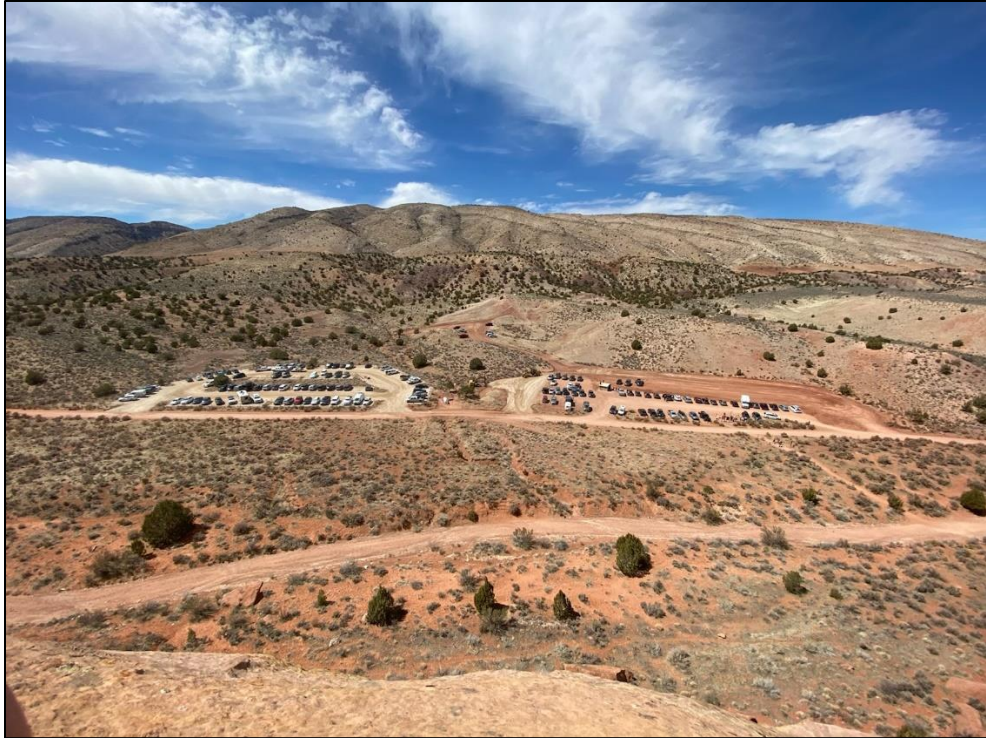
Photo 2: Wire Pass Trailhead expansion project midway through construction. Left parking lot is new. Right parking lot's original footprint is where cars are parked in the photo. Shortly after photo was taken, the right parking lot was completed.
