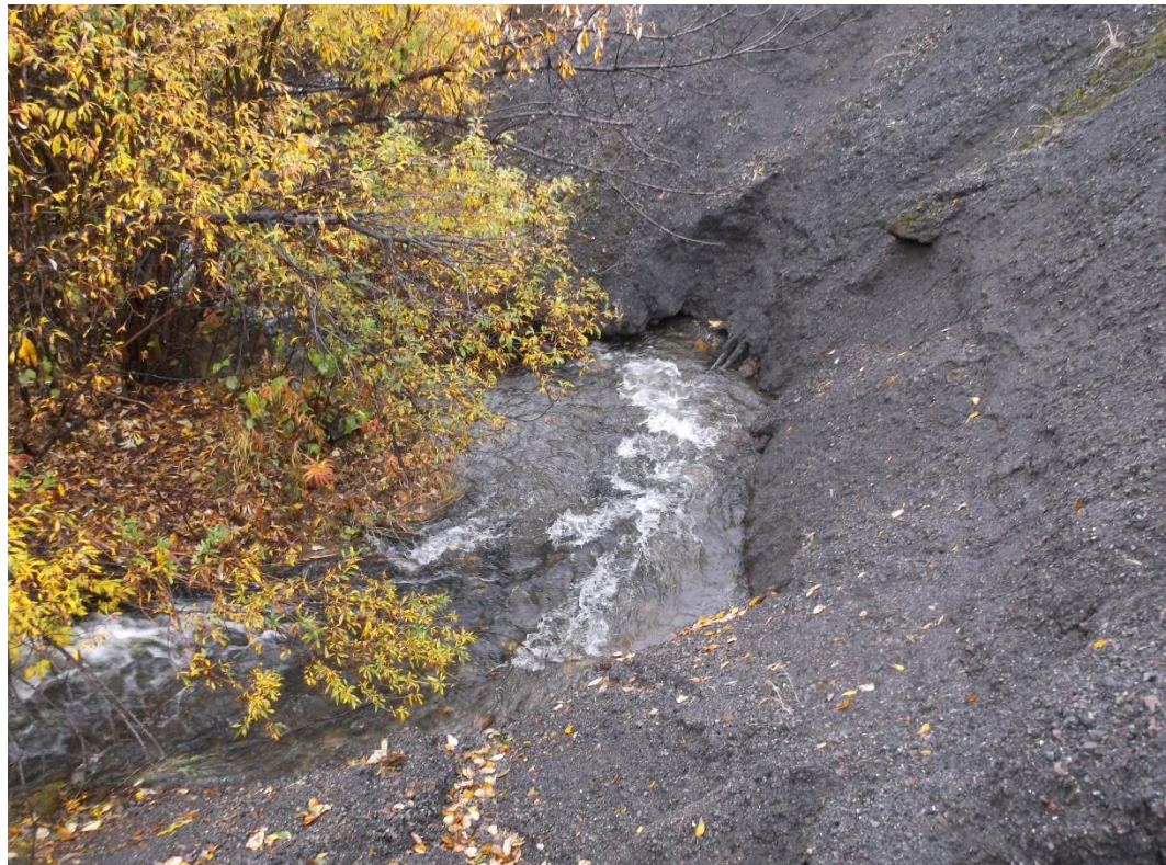
Tailings erosion into Red Devil Creek.
