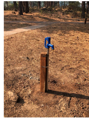
Frost-free hydrant at Topsy Campground
