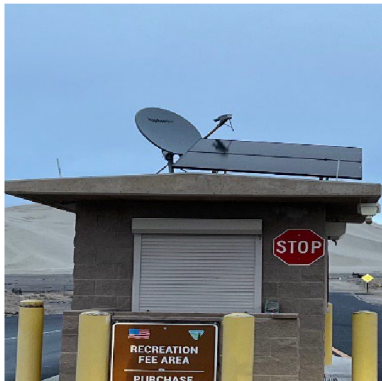
Recently installed Solar/WIFI at Sand Mountain
