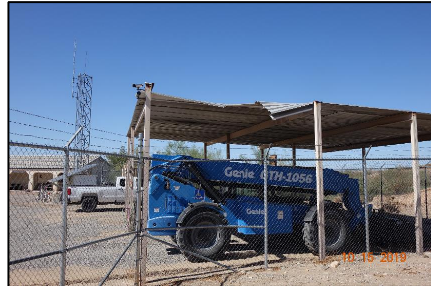
Damaged pole barn roof.
