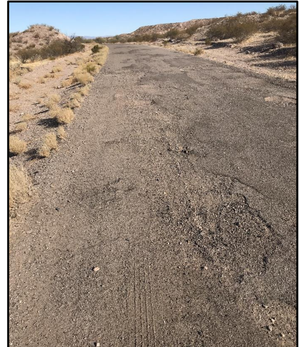
Road is in a failed condition.
