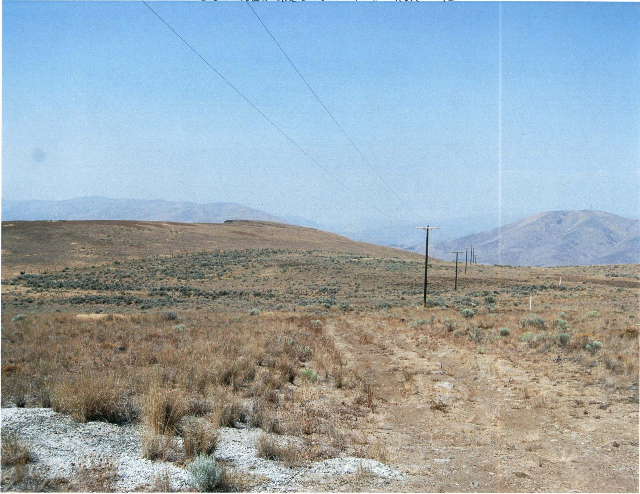
Frame 3: Power line from Communication Site
