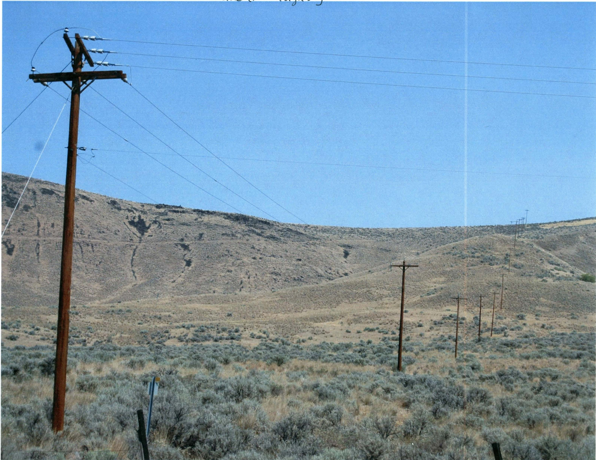
Frame 2: Power line from Highway
