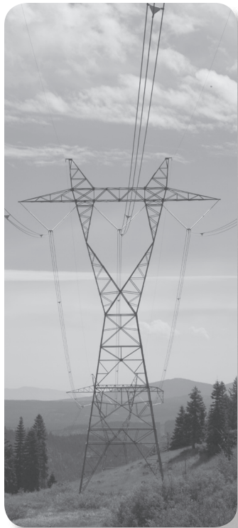
Powerlines on Chinquapin Mountain.
