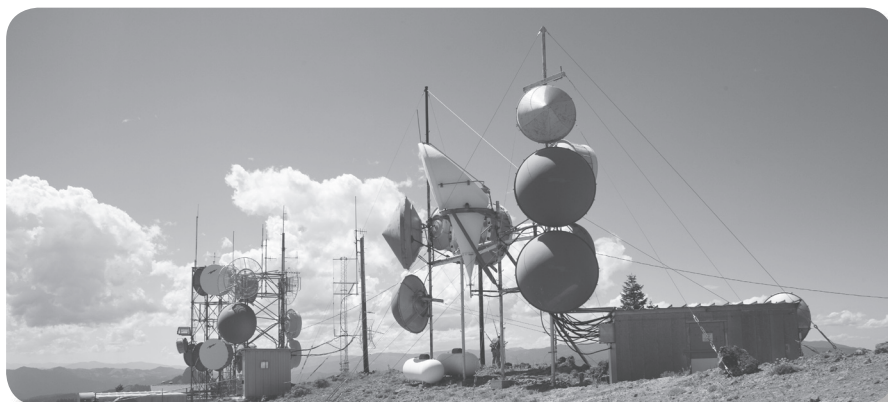
Soda Mountain Communication Site.
