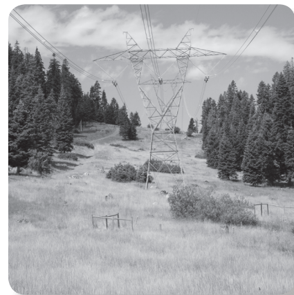
Powerlines on Chinquapin Mountain.
