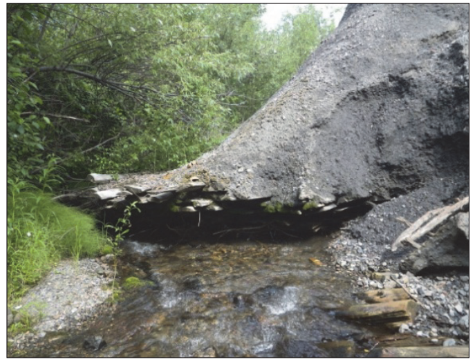
Collapsed bridge and mine tailings at Red Devil Creek
